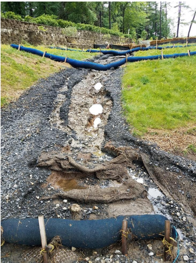
Figure 2. Erosion on lower slope below the vault, July 1, 2020.
