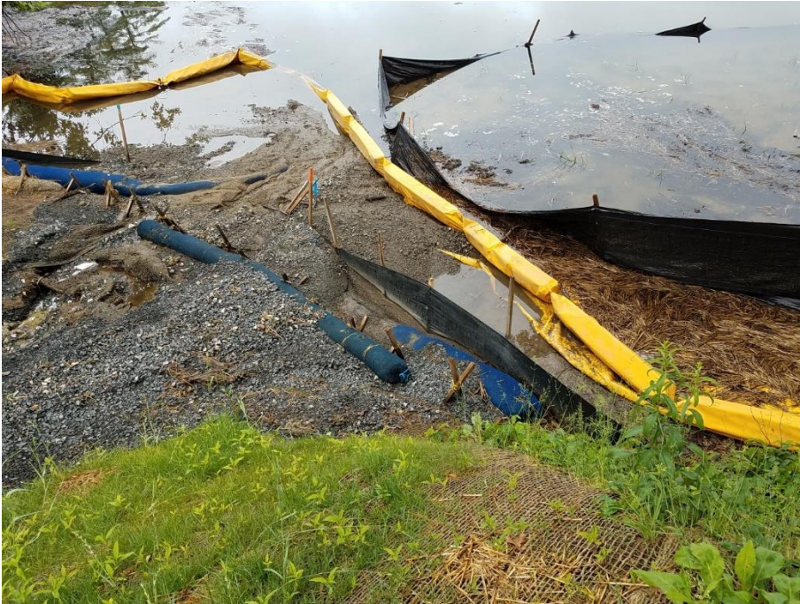
Figure 3. Deposition on tidal flat at toe of slope, July 1, 2020.
