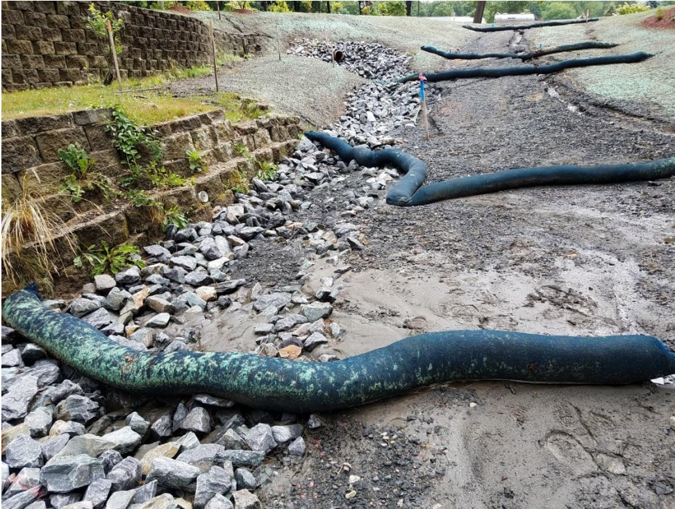
Figure 1. Erosion at top of slope above vault, July 1, 2020.
